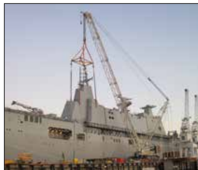
▼ An SyncHoist system used to align steel blocks of the ship's control tower sections allowing gradual lift ingand positioning of the load.
